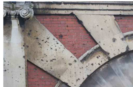
Figure 4: Detail of shrapnel damage from WWII bomb, which exploded outside the Curzon, 4 Jan 1941
