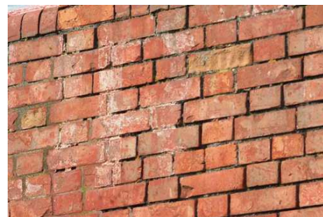
Figure 7: Eroding paintwork –you can just make out the letter 'R' of 'Picture House'
